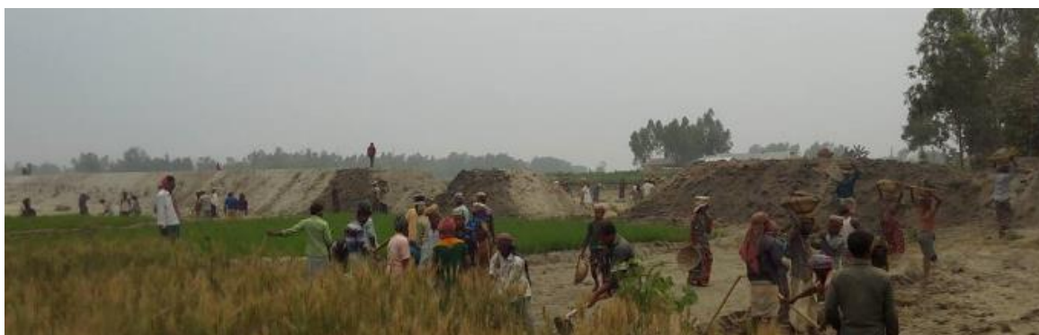
Under cash for work activities, a rural road was constructed in Sapdhori Community, (Photo: Kamrul Hasan/ BDRCS)
