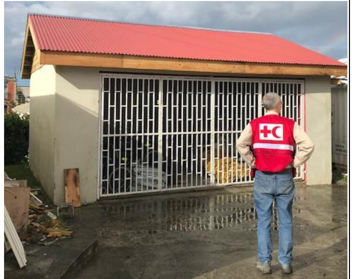
One of the storage units' roof repaired at the NS Headquarters. Source: IFRC
