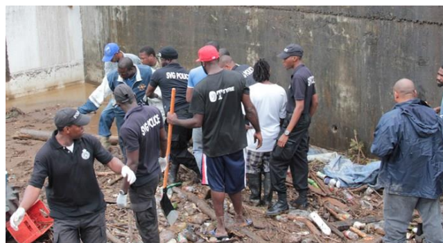
Crews removing debris from a main road in Sandy Bay. Source: SVGRCS
