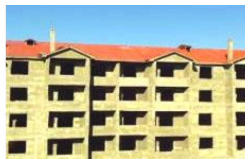
DPRK RCS supported CGI sheets used for permanent shelter roofing in Hoeryong city, North Hamgyong Province in November 2017, (Photo: IFRC and, DPRK RCS)
