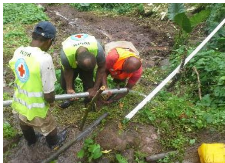
Fiji Red Cross Society branch and community members build a safe water supply in the Tuatua Village in Koro Island. January 2017. (Photo: FRCS)
