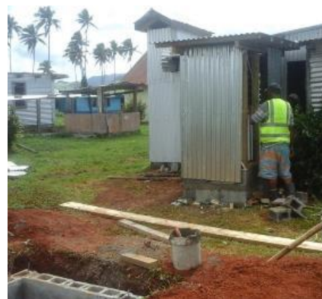
Fiji Red Cross Society and community members constructing a single household latrine in Ra, April 2017. (Photo: FRCS)
