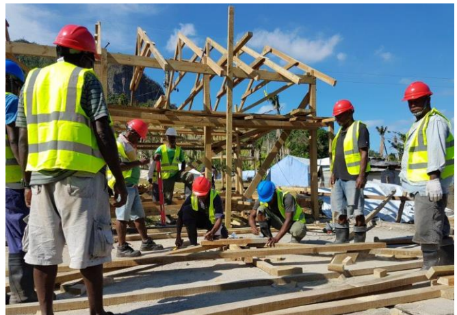
Fiji Red Cross Society and IFRC built model houses and taught villagers how to build back safer. (Photo: Paul Grierson/IFRC)
