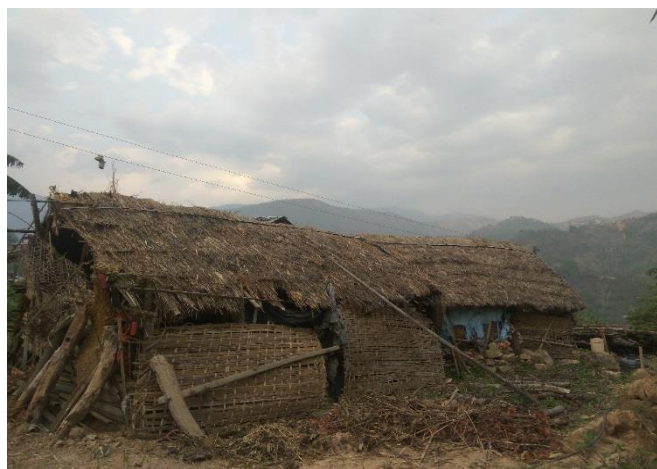
Before: shed in which Toyanath Parajuli's family was living in until Red Cross supported them with shelter cash grants and technical support. (Photo source: NRCS Okhaldhunga District Chapter)
