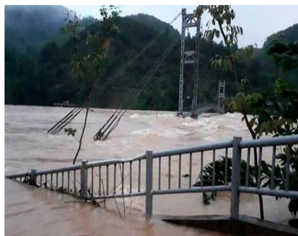
Figure 2: A suspension Bridge in Xuan Cam, Thuong Xuan district of Thanh Hoa was destroyed. (Photo by VNRC)
