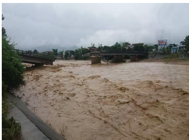
Figure 1: Broken Thia Bridge in Nghia Lo, Yen Bai. (Photo by VNRC)
