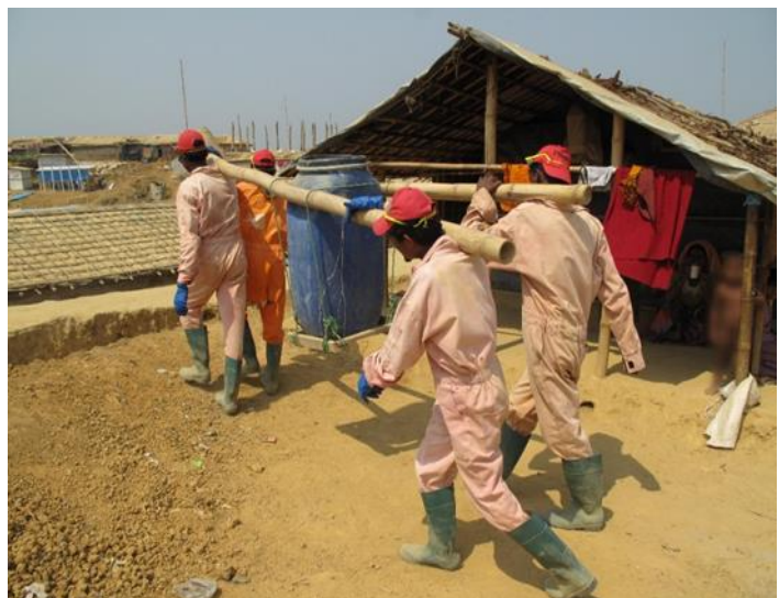
Balukhali 2 Camp (camp 18, Zone XX), Cox's Bazar, Bangladesh, 1 April 2018. Water and sanitation teams of the Red Cross and Red Crescent are preparing for the coming monsoon and cyclone season.
