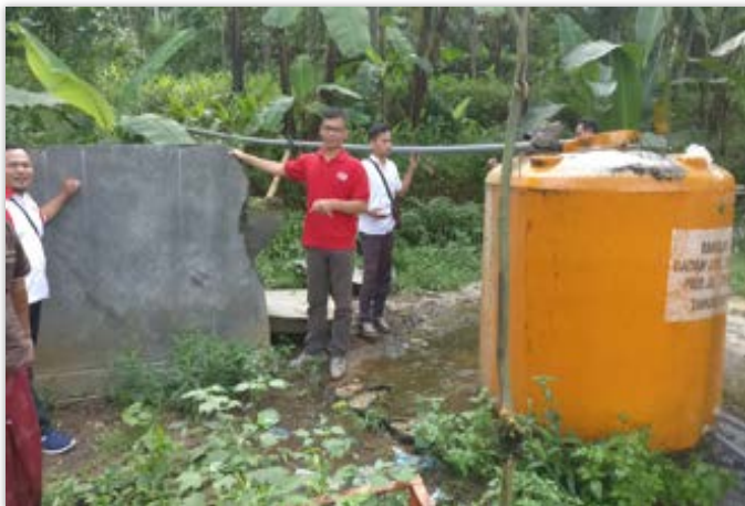
Figure 7 - Temporary repair to broken distribution tank linking a Red Cross pipe to Government water distribution system in Lumajang district, East Java with IFRC evaluation team member, Agung Lestyawan
