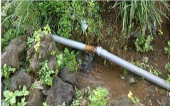
Figure 8 - Local Bamboo repair to detached pipe in Blitar district, East Java
