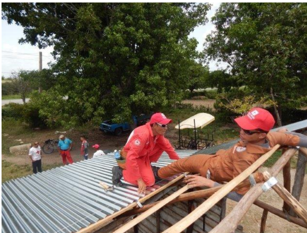
Cuban Red Cross Roofing brigade in the province of Holguin / Source: Cuban Red Cross
