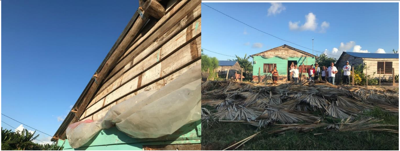
Photographic evidence of properly installed zinc sheets and roof kits in the province of Camaguey / Source: IFRC
