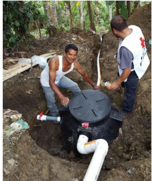
The ERC installed biodigesters in targeted communities. Source: ERC.
