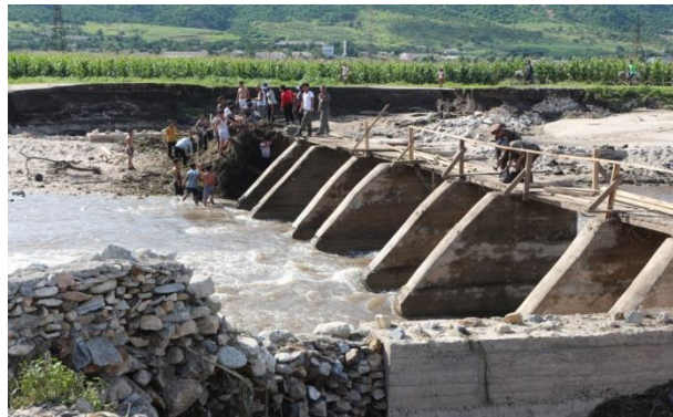
Damaged water dam. (Photo: DPRK RCS)
