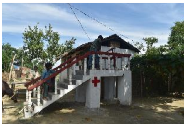
An elevated tube-well was constructed in Rajpur Municipality, Ward No.1, Rautahat district. Laxmi Ram said "we used to drink water of 30/35 feet deep and it was not safe to drink, but now we are drinking safe water of 245 feet deep. Water quality was tested and is potable to drink". (Photo credit: NRCS)
