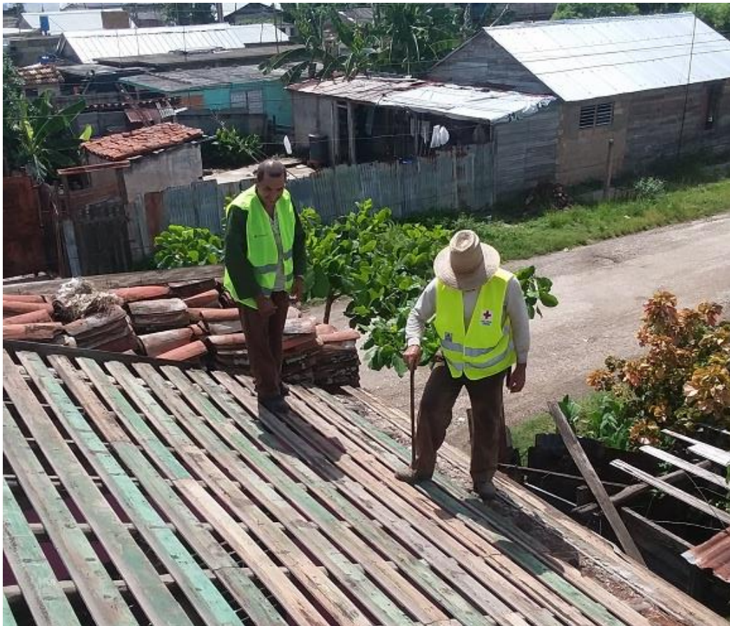
Cuban Red Cross Roofing brigade in the province of Camagüey/ Source: CRC
