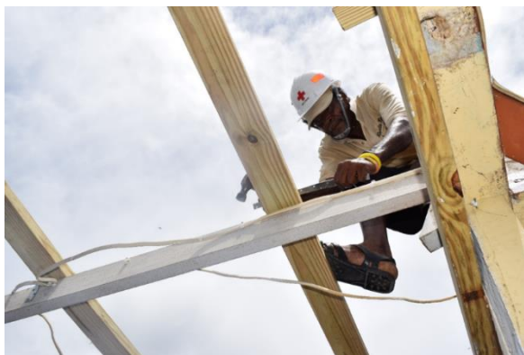
Left and right: Damaged roofs undergoing repair work in Dominica. Source: DRCS.
