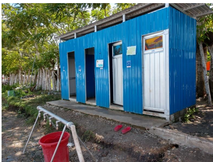
Latrines and bathing cubicles constructed in Gunung Bale IDP camp. (Photo: IFRC)
