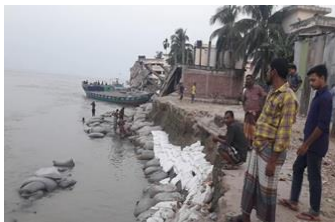
Residents observing the impact of the riverbank erosion in Shariatpur district. The collapse of embankments caused destruction of farmlands, houses and infrastructures situated along the affected stretch of the river. (Photo: IFRC)
