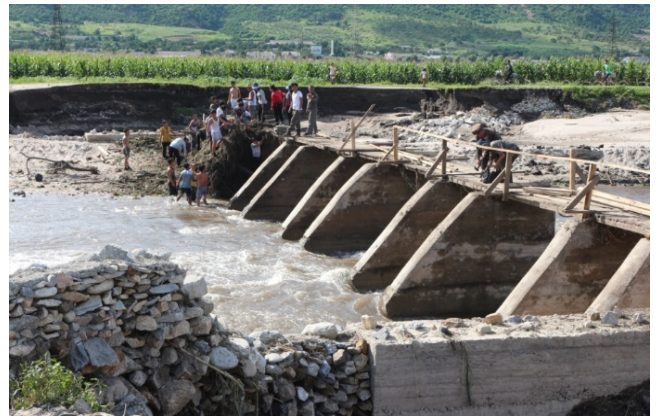
Damaged water dam. (Photo: DPRK RCS)
