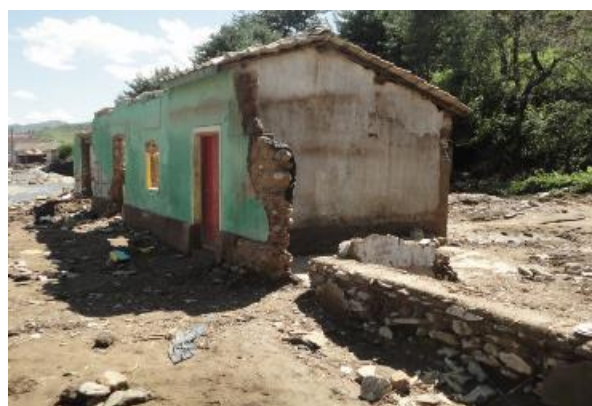
Significant damage to Houses in Eup Town, Jangpung County (Photo: John Fleming/IFRC)
