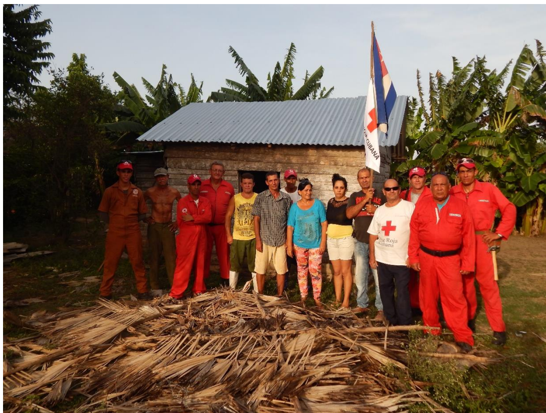
Cuban Red Cross Roofing brigade after the installation of a roof/ Source: CRC
