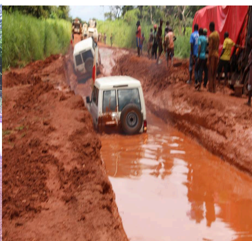
Example of poor road conditions ©CAR RC
