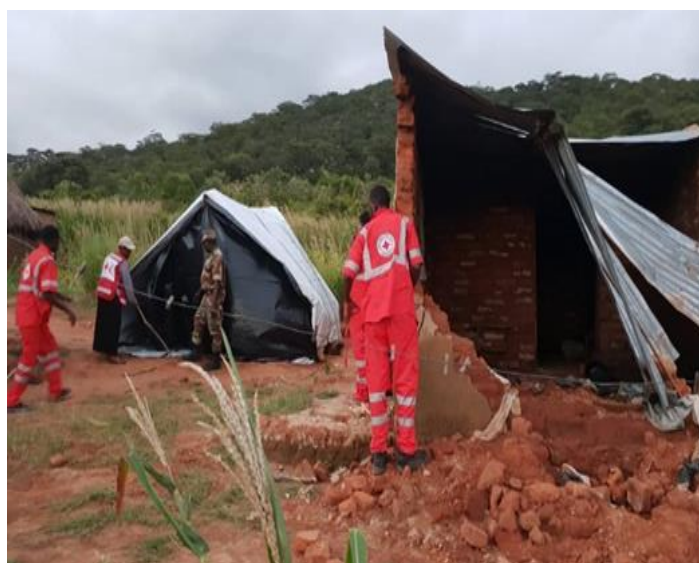
ZRCS response team members constructing emergency shelter for a family affected by Tropical Cyclone Idai in Masvingo Province ©ZRCS
