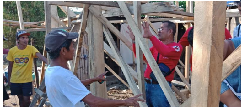
Shelter team working with carpenters and community households on the first pilot shelters in Cagayan. (Photo: PRC)
