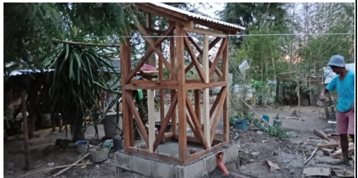
Ongoing latrine superstructure construction in barangay Afusing Daga, Alcala, Cagayan Valley. (Photo: PRC)
