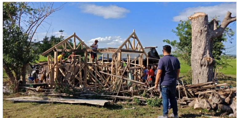
Shelter team working with carpenters and community households on the first pilot shelters in Cagayan. (Photo: PRC)
