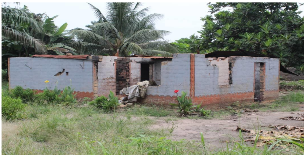
Example of a house destroyed during clashes between Nunu and Tende
