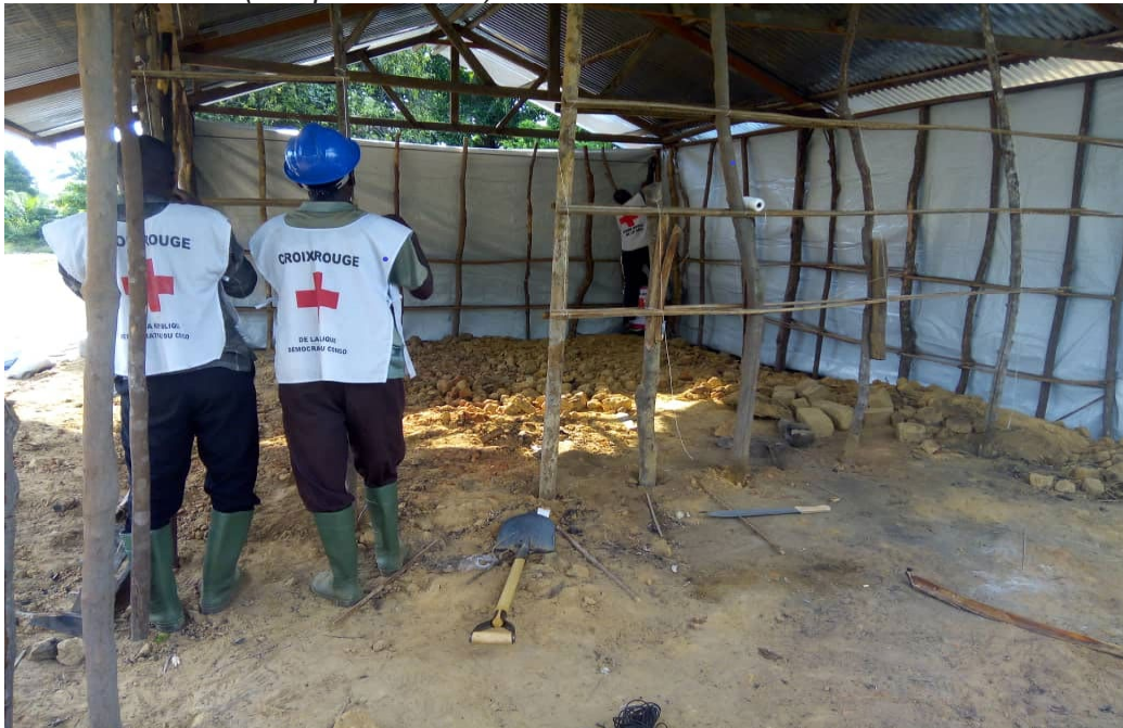
These Volunteers of the DRC RC are completing the construction of a shelter tolerated by the Military Genie
