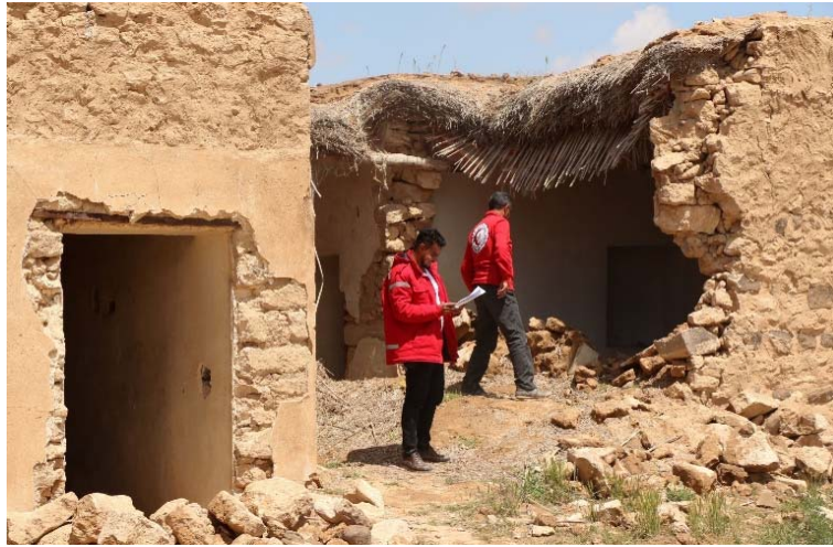
SARC volunteers assess damaged houses in Tal-Hamis.
