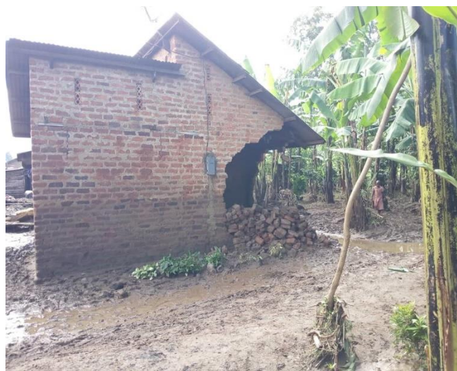
A house destroyed by floods disaster in Sironko district
