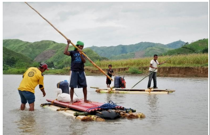
Shelter beneficiaries used a raft made from banana stem to haul the CGI sheets from the main drop off point to the relocation site. (Photo: PRC/IFRC)
