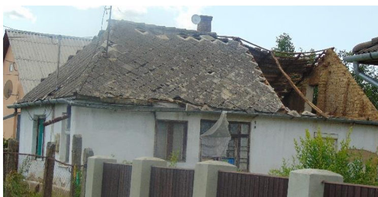
Image 1: One of the 2,400 private homes that were damaged in the storm on 17 June. Photo: HRC
