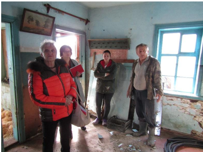
Image 3. A man is showing the damages inside of his house in Apsheronsk to the representatives of Krasnodar Krai Red Cross branch, IFRC and local administration. Photo by IFRC
