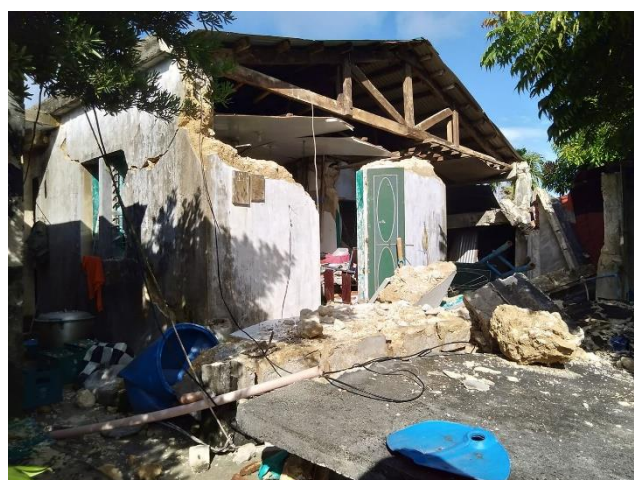
Some shelters are damaged after the earthquake struck Itbayat, Batanes. PRC team continue to assess the damage in the area. (Photo: PRC)
