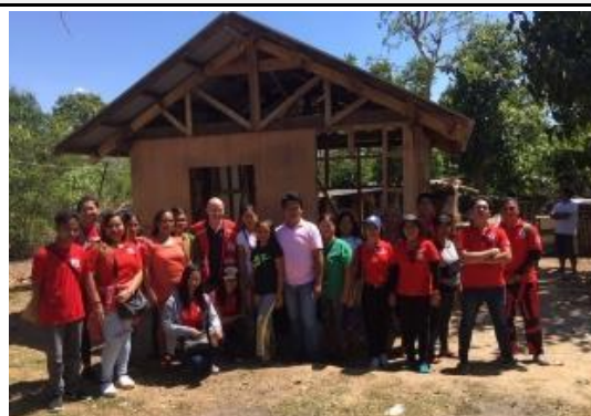
Shelter volunteers and chapter staff who have been mobilized and trained on the build back safer techniques. (Photo: PRC)
