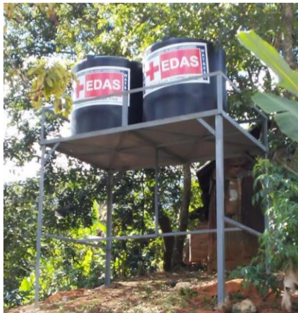
Photo 8: Tanks for the distribution system – El Maniel Source: DRC 2018.
