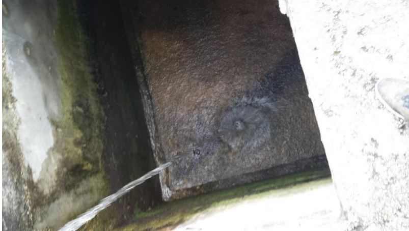
Photo 7: Cistern in poor condition and unsuitable for water collection - El Maniel. Source: DRC 2018.
