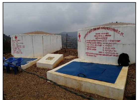
Image 3. Water lifting schemes utilise a series of 'pump and tank stations' to pump water to communities located above water sources. The NRCS highest water lifting scheme constructed lifts water 940 meters from source to community supply. Pictured are the two 20,000 litre water tanks, Danda Tol village.
