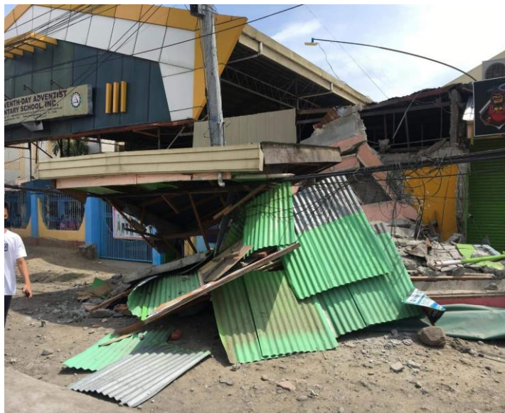
Some of the infrastructure were damage by the earthquake including schools and public buildings on 29 October 2019. (Photo: PRC)
