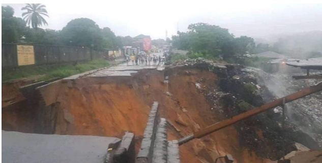
Road destroyed by the flood water. Photos DRC RC Volunteers
