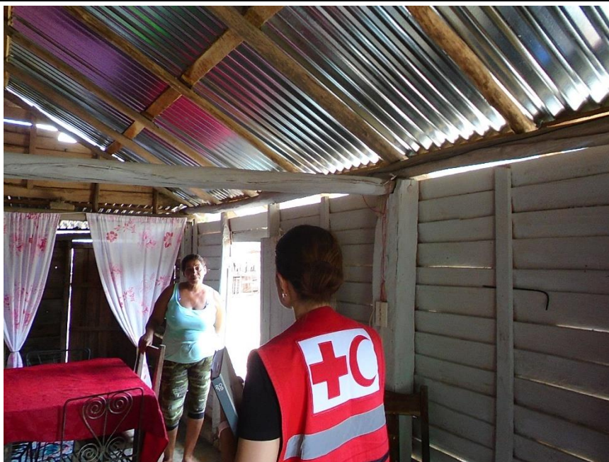
Photo 2: IFRC monitoring visit of the repaired roofs in the Minas Community, Camagüey, Municipality. Source: IFRC 2019.
