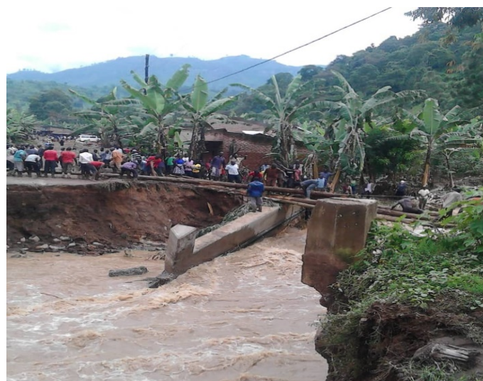
Collapsed bridge resulting from floods and landslides in Bududa district ©URCS
