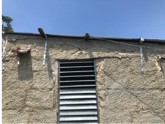
Photo: Incorrect use of anti-hurricane tape.
