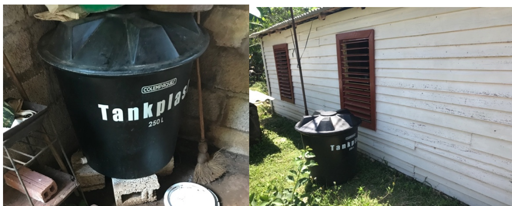
Photo: Water tanks.
