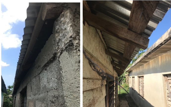
Photos: Houses without proper installation (nails have not been bent).
