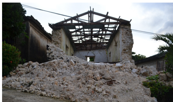
Earthquake impact on houses at Itbayat. (Photo: PRC)
