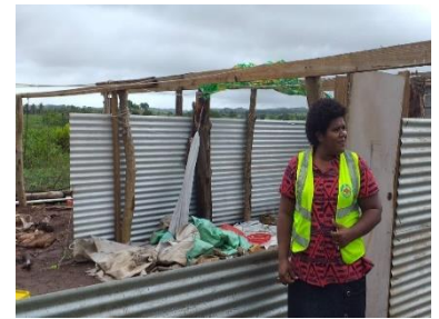
Volunteers assessing damage houses in Ba. (Photos: FRCS)
