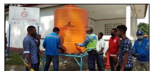
Installation of water tank for a handwashing facility in Dili. (Photo: CVTL)
