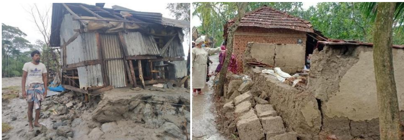
Left - A resident inspects his damaged house due to tidal surge and heavy wind in Bagerhat (Photo: IFRC/AmCross); Right - One of the many collapsed houses in Satkhira (Photo: BDRCS)
