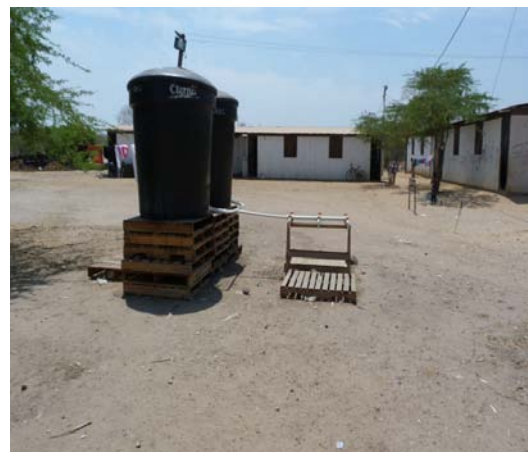
Water distribution point installed in La Candelaria municipality. Source: CRCS
