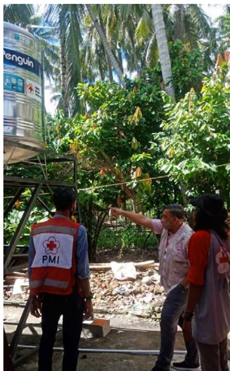
One of the water tanks and water towers installed in the target communities aimed at ensuring adequate supply of water for household use. (Photo: IFRC/PMI)
