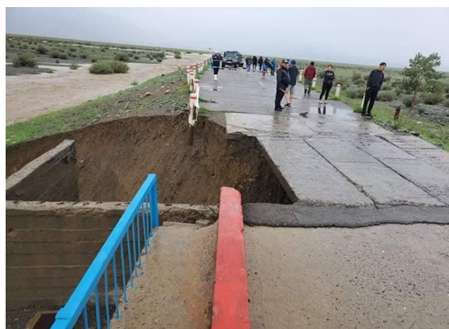
Damaged bridge in Uvs province. (Photo: MRCS)
