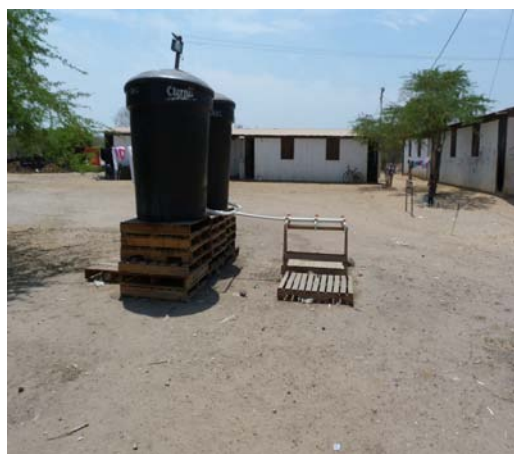
Water distribution point installed in La Candelaria municipality. Source: CRCS
