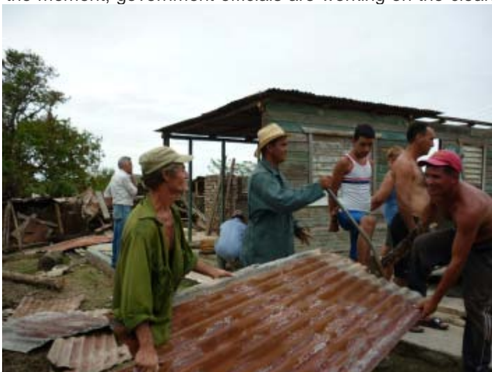
Community members are helping out with some fast repairs to the home of a 77 year old man that lost his home after the passage of hurricane Sandy. Source: IFRC
