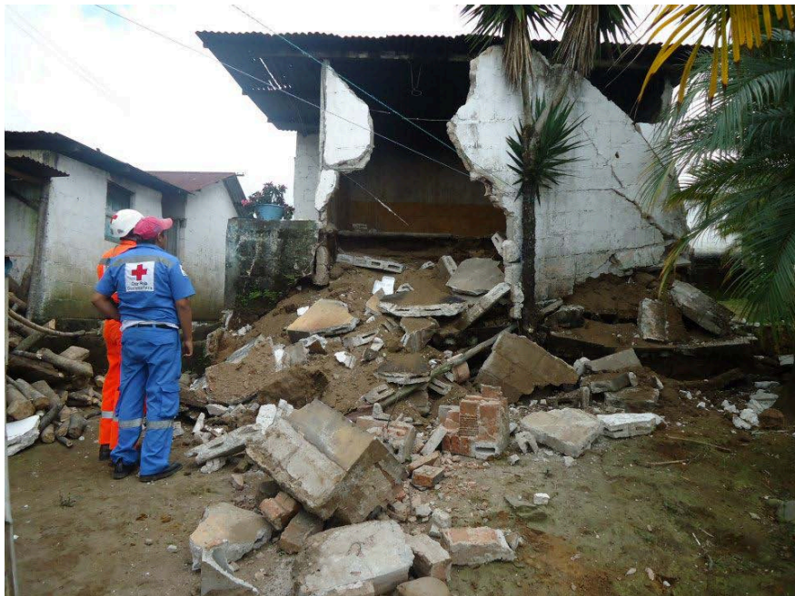
On 7 November a 7.4 magnitude earthquake was felt in Guatemala, affecting several areas, in particular San Marcos where several buildings collapsed. Source: Guatemalan Red Cross
