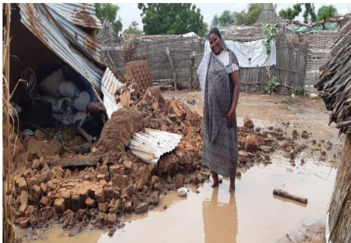
Affected resident in South Darfur State standing on the rubbles of her destroyed home ©SRCS
